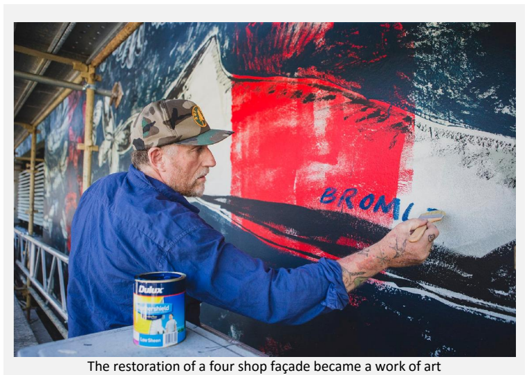
The restoration of a four shop façade became a work of art
